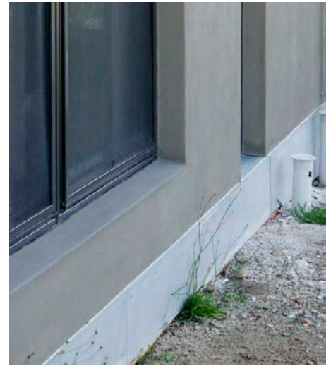
↑ Newly completed slab edge including insulation and termite barrier using the ISEG.2 approach.
