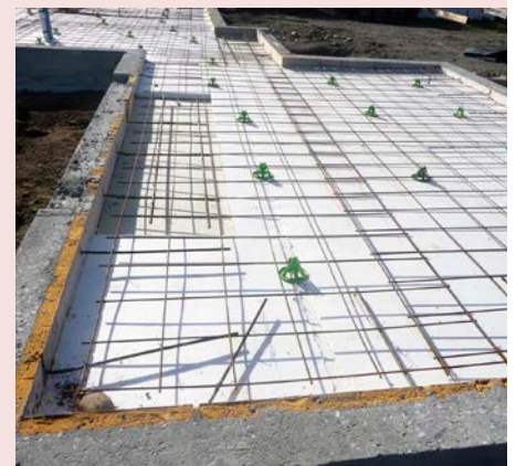
↑ Regular slabs can be fully insulated as well, and there’s a range of foam products designed specifically for under-slab use.
